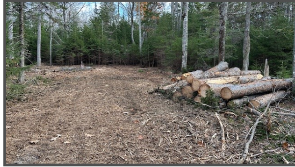
One of the test boring sites which are cleared to a 25 foot radius around the drilling location.
