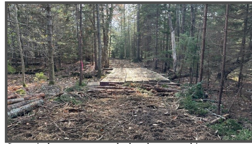
Large timber mats are used when heavy machinery crosses a stream or wetland area.
